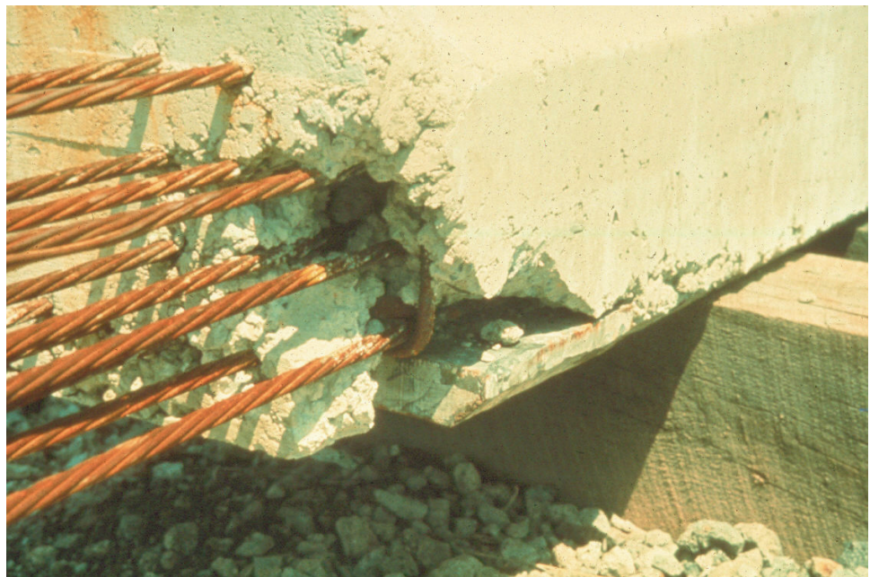
Figure 7.9.10 Spalling Due to Poor Concrete
