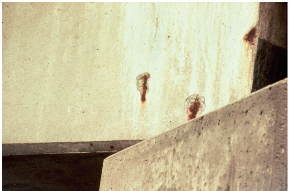
Figure 7.10.12 Exposed Bars at End of Box Beam
