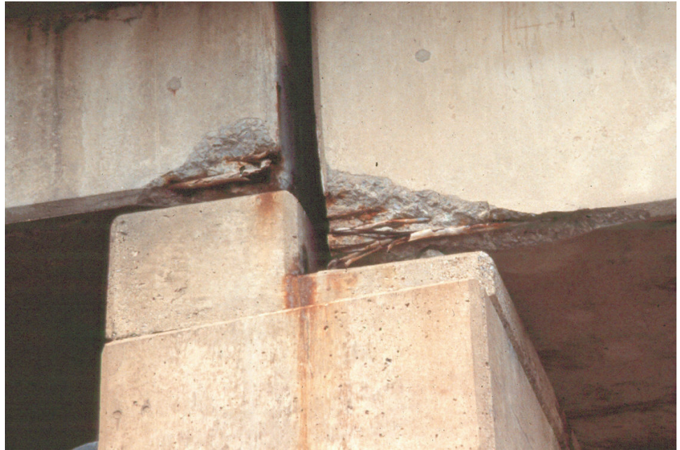
Figure 7.10.11 Spalled Beam Ends
