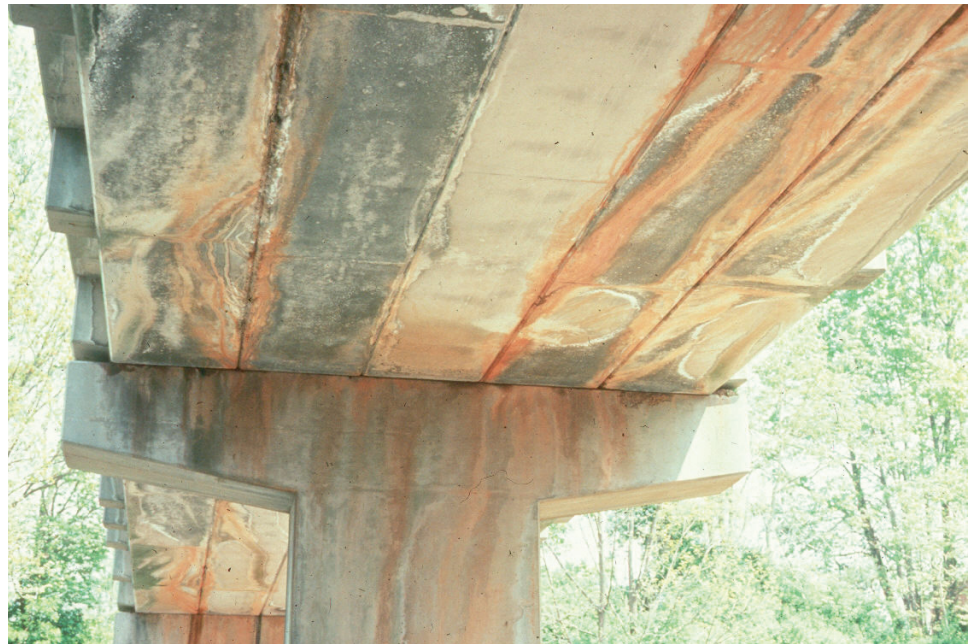
Figure 7.10.16 Joint Leakage and Rust Stain
