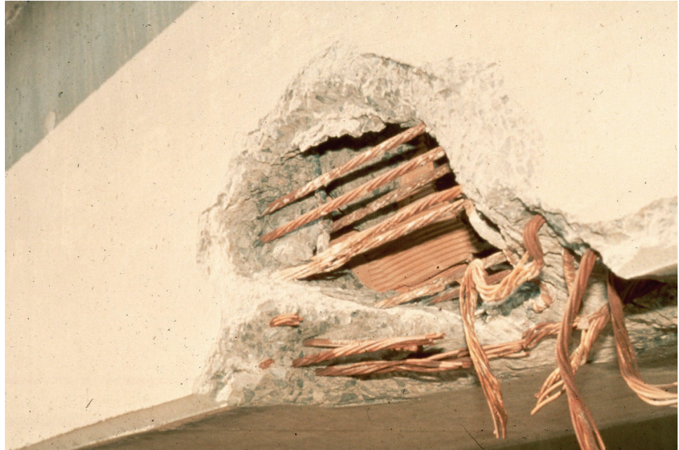
Figure 7.10.17 Close-up of Collision Damage
