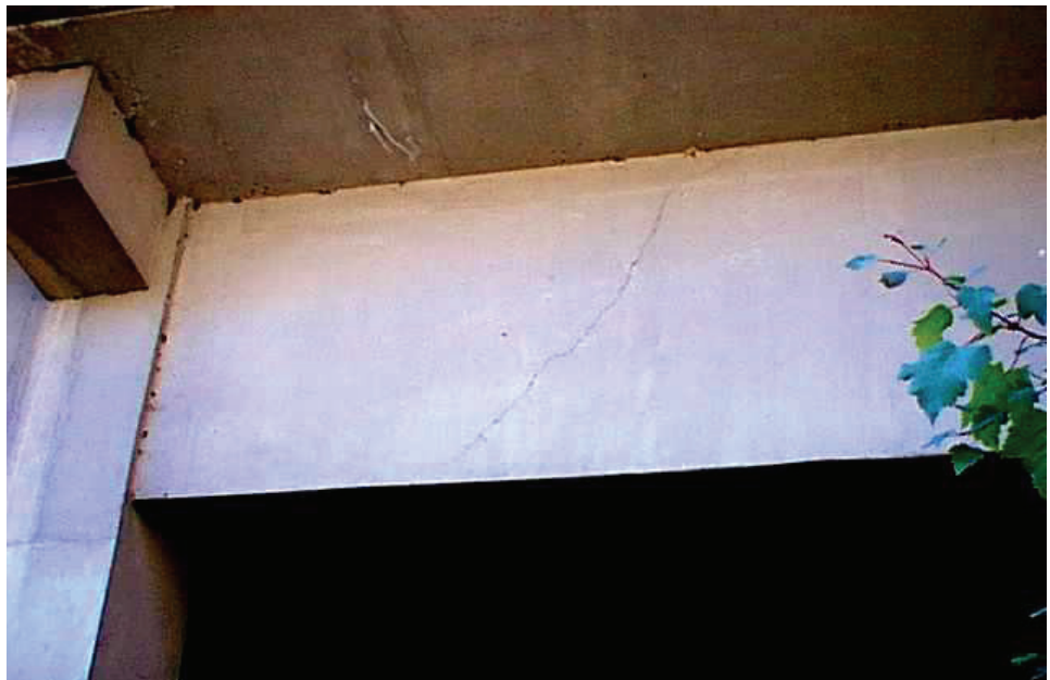
Figure 7.10.14 Diagonal Shear Crack in Web of Beam
