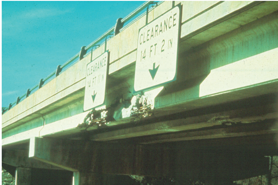
Figure 7.9.14 Collision Damage on Prestressed Concrete I-beam
