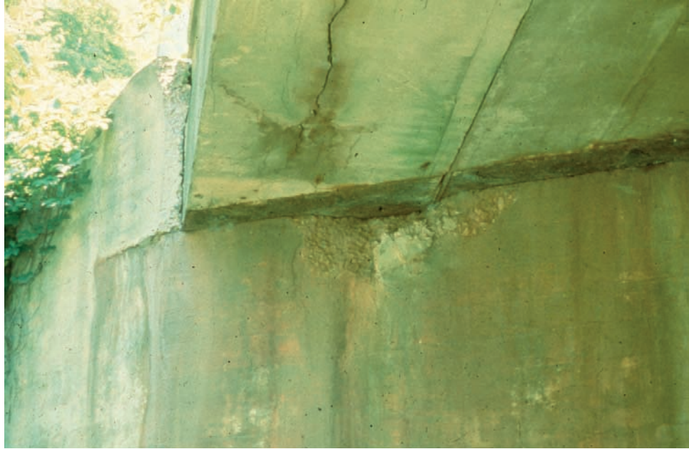
Figure 7.10.13 Longitudinal Cracks in Bottom Flange of Beam
