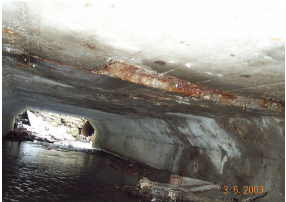
Figure 7.12.10 Spalls and Delaminations
