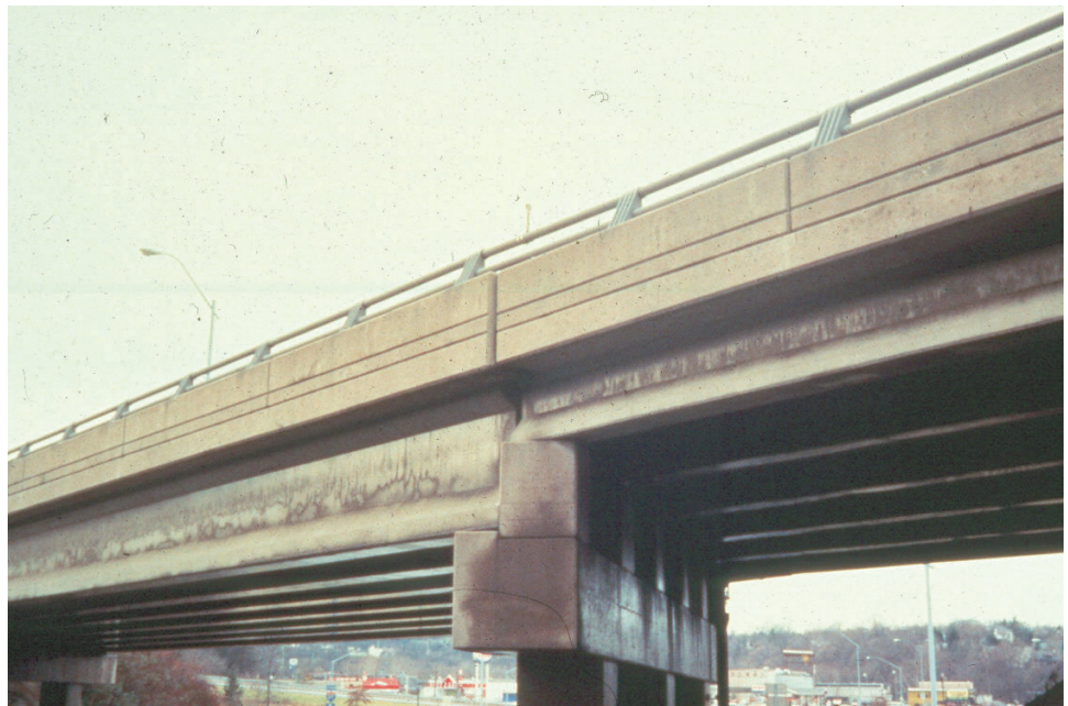
Figure 7.9.13 Leakage of Water at Joint between Spans
