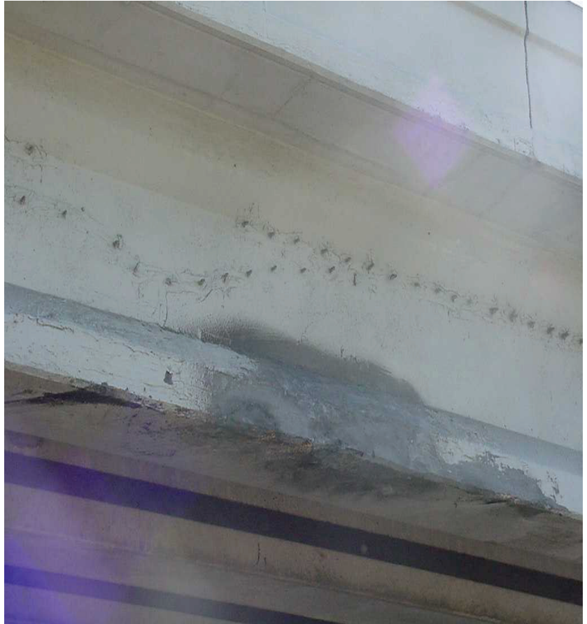
Figure 7.9.15 Collision Damage Repair on Prestressed Concrete I-bBeam. Note Epoxy Injection Ports
